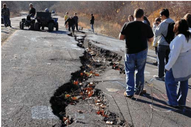
Fig. 5. Damage to Rt. 61 from underground mine fire; Centralia, PA; 11-15-10. Centralia's population has dwindled from 1000+ residents in 1981 to 7 in 2010 as a result of mine fire burning beneath the borough since 1962. In 1992, the Commonwealth of PA condemned all properties under eminent domain. A few residents remain in spite of a failed lawsuit to reverse the decision. Several current and former Centralia residents believe the state's eminent domain claim was a plot to gain the mineral rights to the anthracite coal beneath the borough. For two decades following the start of the fire, the mines were flushed with water and fly ash (pozolone mixture that sets up like cement), excavated the burning material and dug trenches, backfilled, drilled again and again in an attempt to find the boundaries of the fire and to put it out. By the early 1980s the fire had affected approximately 200 acres and homes had to be abandoned as carbon monoxide levels reached life-threatening levels. An engineering study in 1983 concluded the fire could burn for another century or even more and could spread over 3700 acres.
