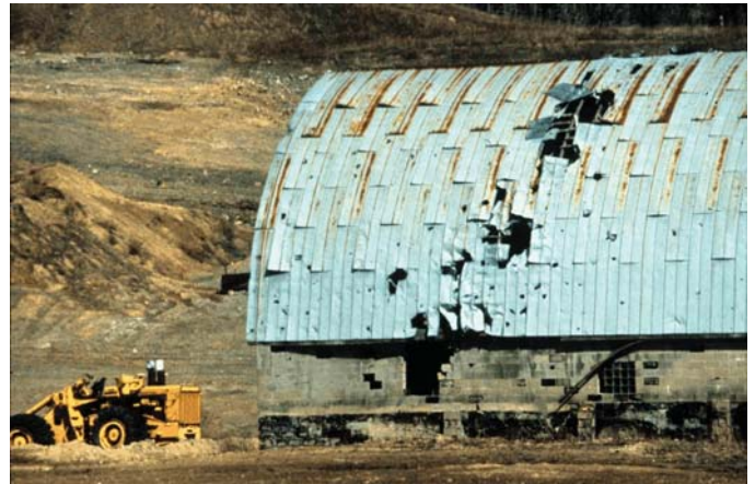
Damage from fly rock. Blasting at a nearby bituminous strip mine produced fly rock (a.k.a. ejecta material) that damaged this structure.
