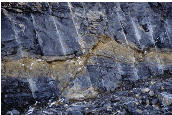
Normal fault in the Gatesburg Formation, exposed during construction of the I-99 Scotia interchange; 12-22-2001. (image by the author)
